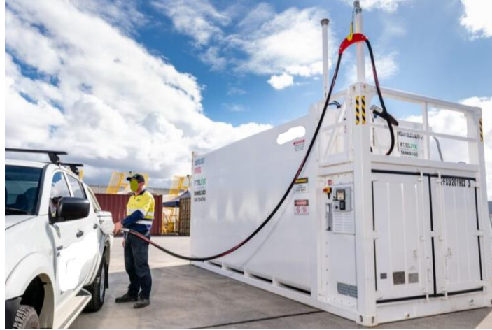
Sample fuel facility - (source www.fuelfix.com.au )
