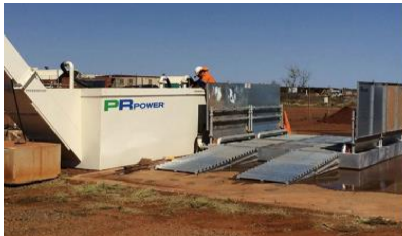
Sample wash facility - (source www.prwater.com.au )
