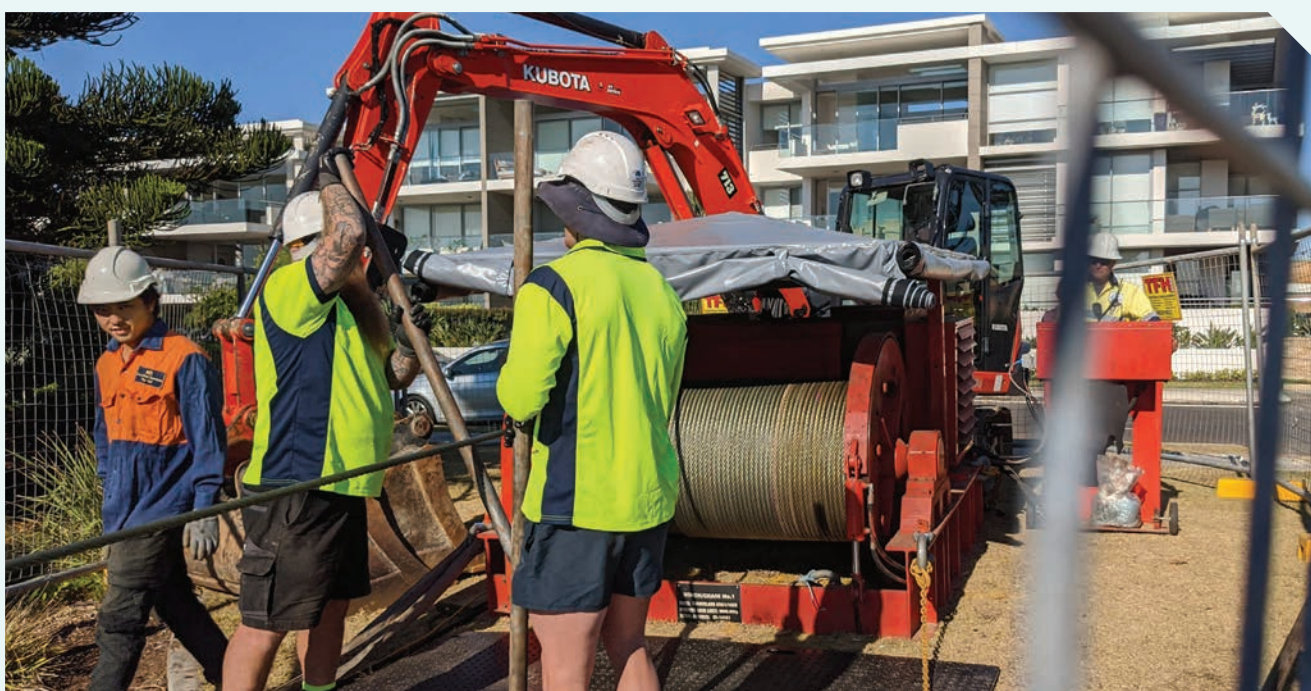
Laying cable (Source: Queensland Capacity Network Pty Ltd, trading as QCN Fibre)
