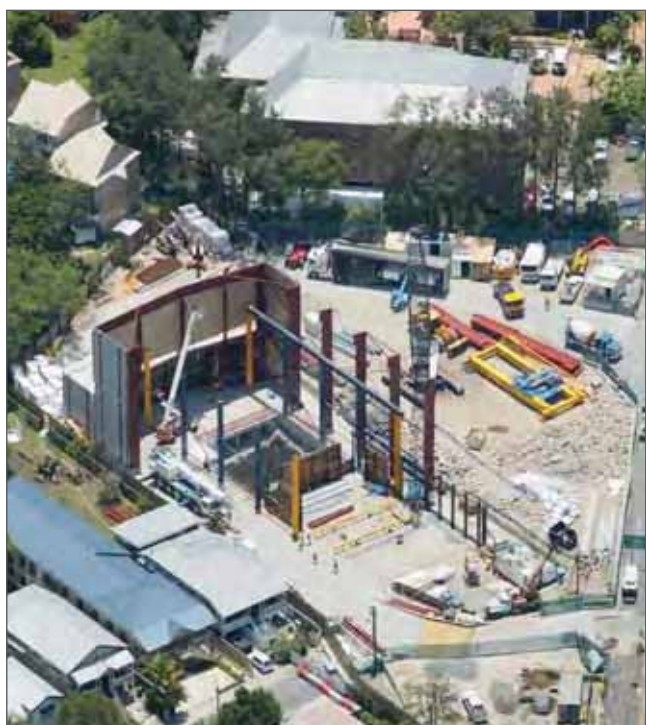
Kangaroo Point workshed, Clem Jones tunnel Photo courtesy of Brisbane City Council
