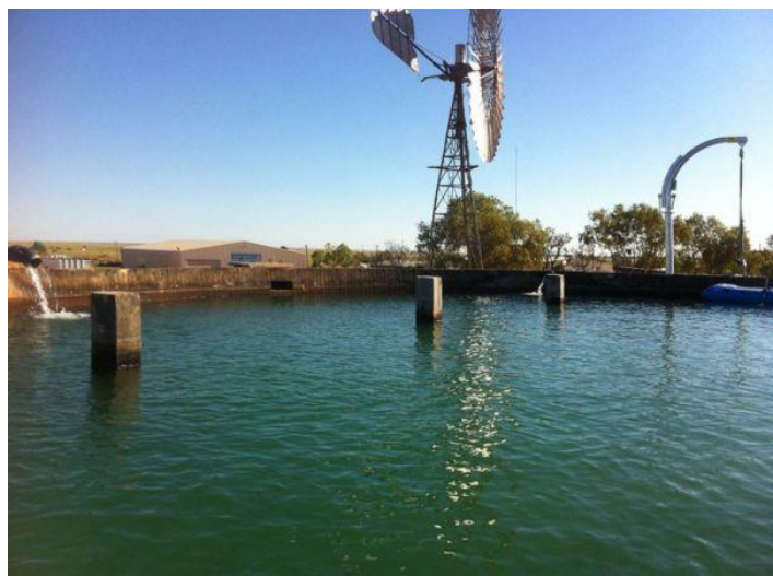
Above: the Boulia Reservoir with the roof removed, ahead of a new and secure covering.
