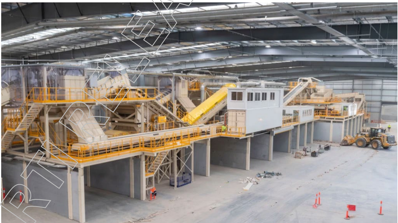
Photo 2: RDF Facility at Wetherill Park (source: ResourceCo)
