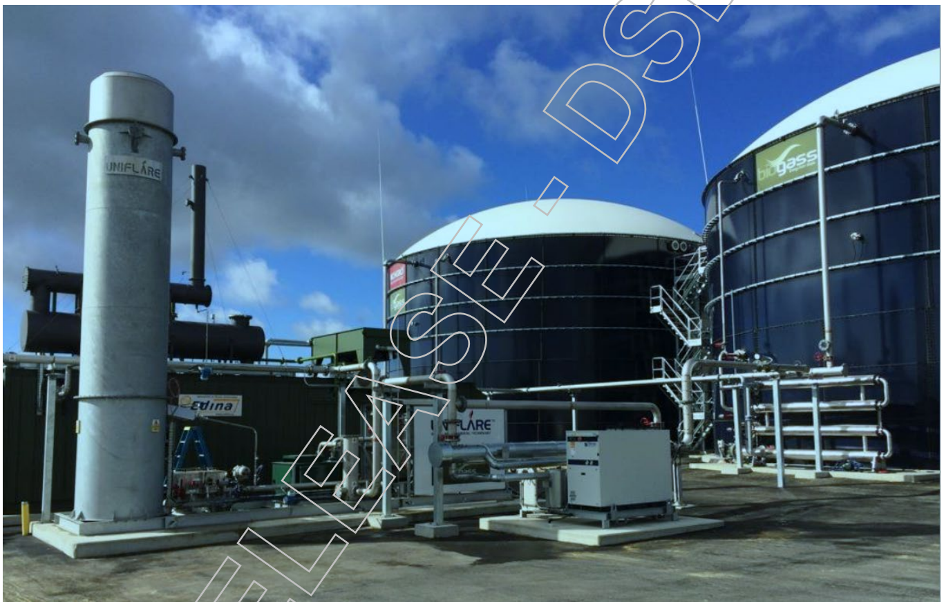
Photo 1: Richgro's anaerobic digestion facility (source: Biogas Renewables)
