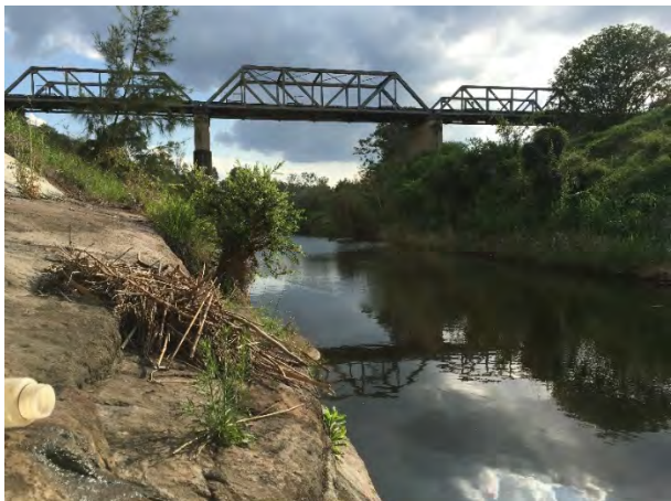
Photograph 4.1 Lockyer Creek at Project alignment waterway crossing displaying absence of aquatic macrophytes (FFJV 2017)
