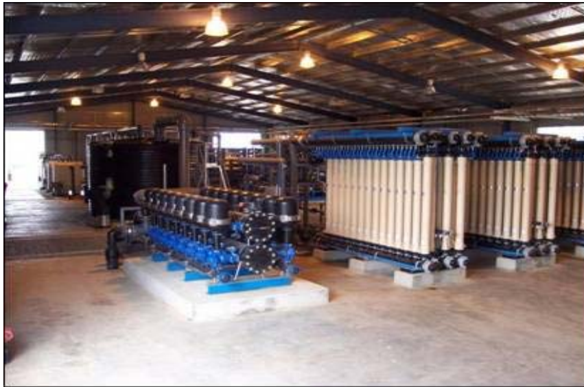
Plate 3 APLNG’s operating reverse osmosis plant at Spring Gully
