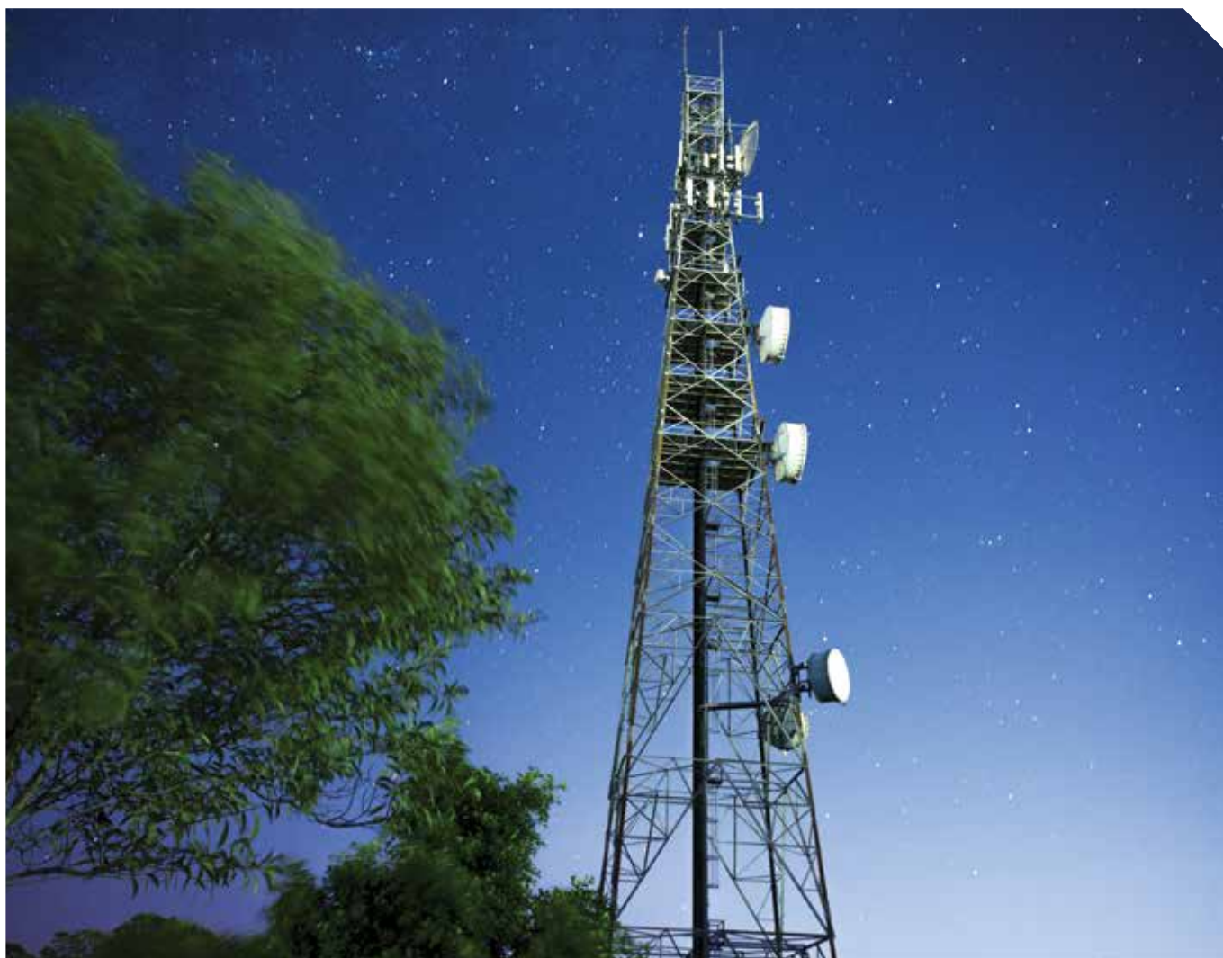
Digital mobile towers
