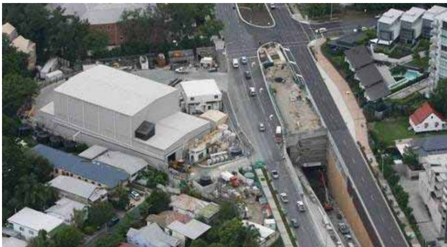
Photo 5-6: Acoustic Shed located at Shaftson Avenue Worksite (CLEM 7)
