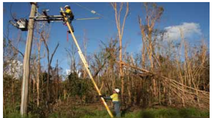
Photo of Ergon Energy workers repairing the network courtesy of Ergon Energy
