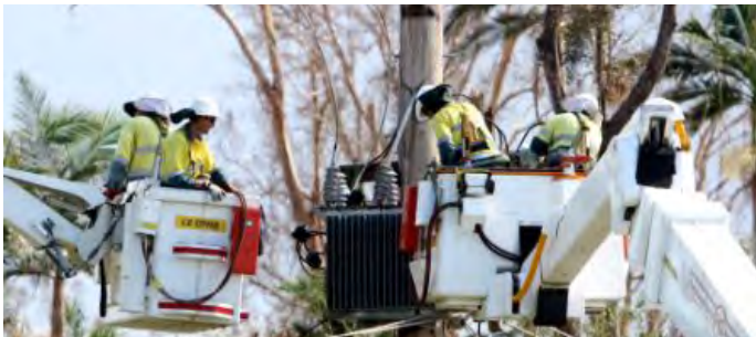
Photo of repair works underway after Cyclone Yasi provided courtesy of Ergon Energy.
