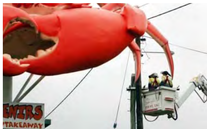
Photo of repairs in Cardwell provided courtesy of Ergon Energy
