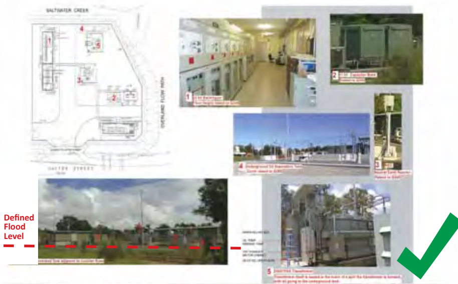
Figure 6: Example of resilient substation design with all sensitive electrical equipment raised above the flood level
