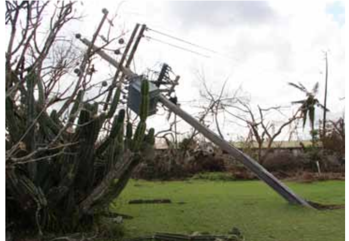
Photo of fallen powerlines at Tully Heads provided courtesy of Queensland Government
