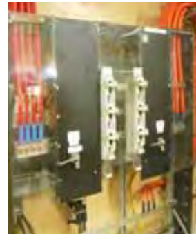
Photo 5: Low voltage switchboard courtesy of Queensland Government
