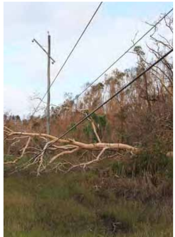
Photo of powerlines damaged by fallen vegetation in Tully Heads, courtesy of Ergon Energy
