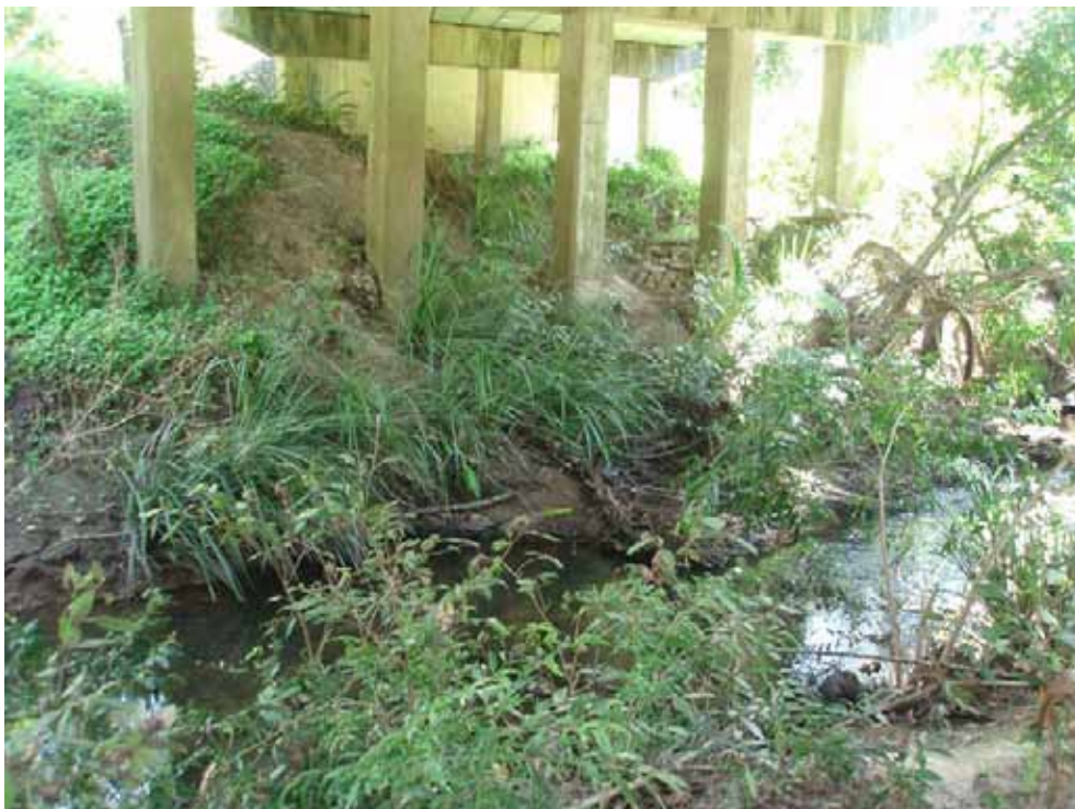
Plate 9: North Maroochy River directly adjacent and downstream of the crossing point (facing south). Southern bank with little or no riparian vegetation under road bridge.
