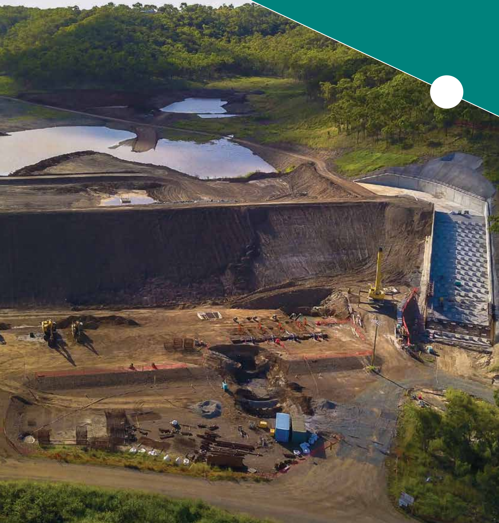
Offline storage and repump station site, Gladstone
