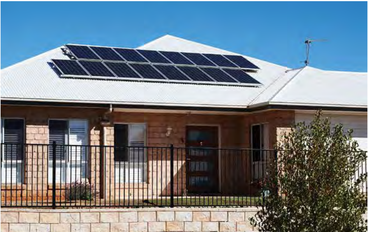
Rooftop solar panels
