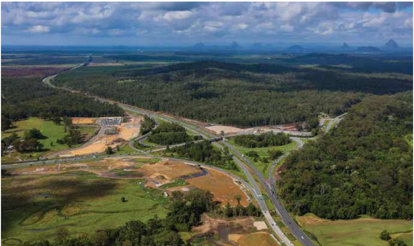
Interchange works on the Bruce Highway at Caloundra Road and Steve Irwin Way
