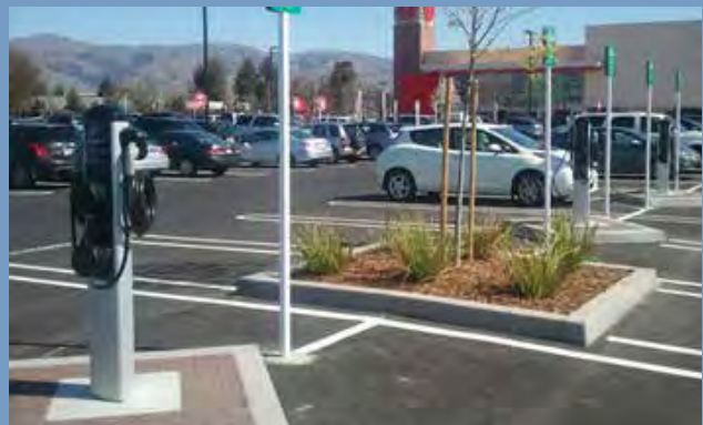
Figure 6. Destination chargers in a large shopping centre carpark
