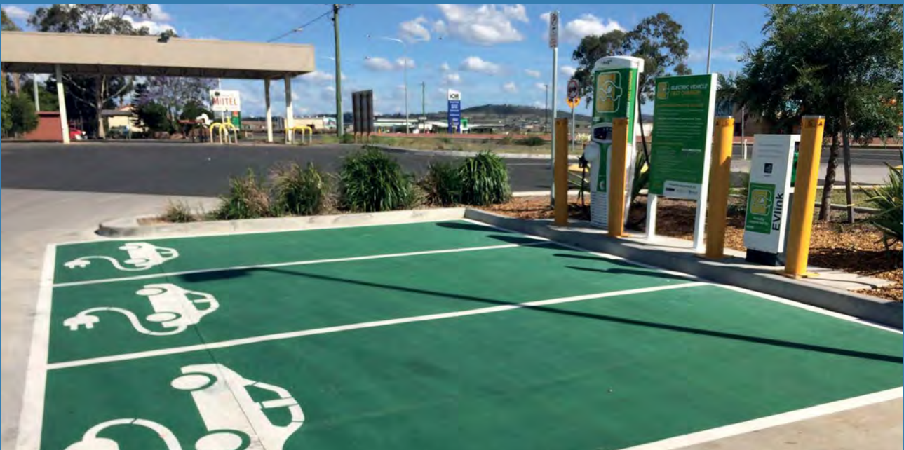
Figure 9. Toowoomba fast charging station on the Queensland Electric Super Highway
