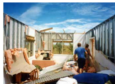
Photo 4 – inadequate roof truss anchorage
