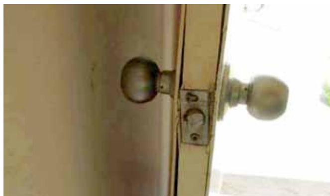
Photo 6 – Damage to door lock after high winds. Source: Cyclone Testing Station, James Cook University.
