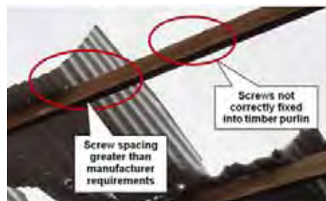
Photo 2 – roofing fasteners not installed in accordance with manufacturer's recommendations
