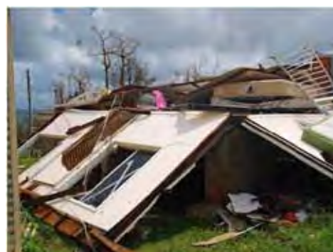
Photo 5 – inadequate tie-down through the entire structure
