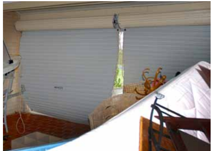
Photo 7 – Roller doors damaged after being hit by high winds. Source: Cyclone Testing Station, James Cook University.
