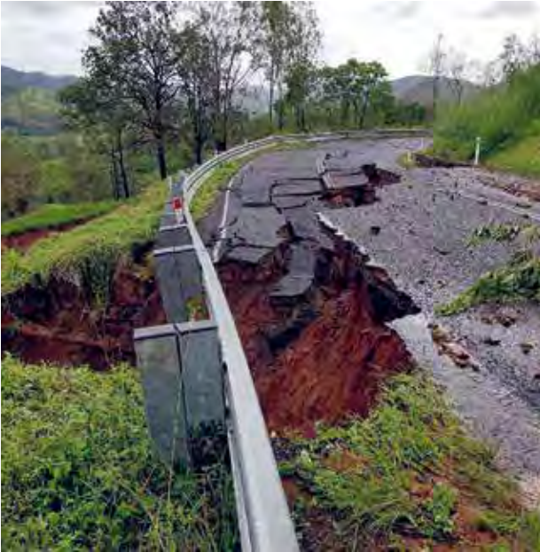
Severe Tropical Cyclone Debbie caused severe damage on the Sarina Range crossing
