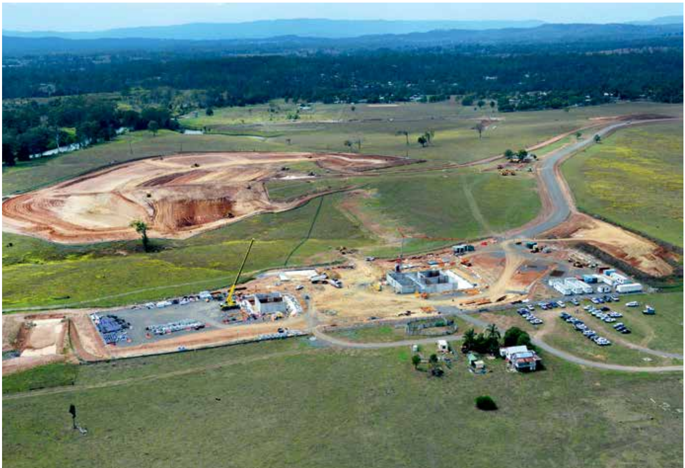
Cedar Grove Wastewater Treatment Plant
