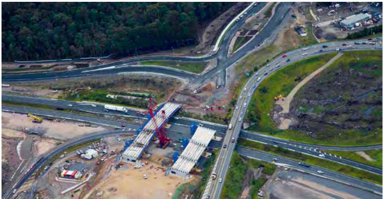
The construction of the diverging diamond intersection at the Caloundra Road turn-off on the Bruce Highway on the Sunshine Coast
