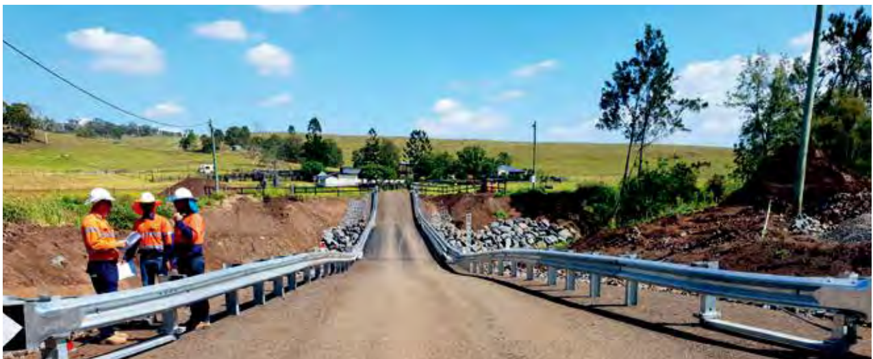
Haack Bridge in the Scenic Rim required extensive reconstruction works after it was damaged by Severe Tropical Cyclone Debbie
